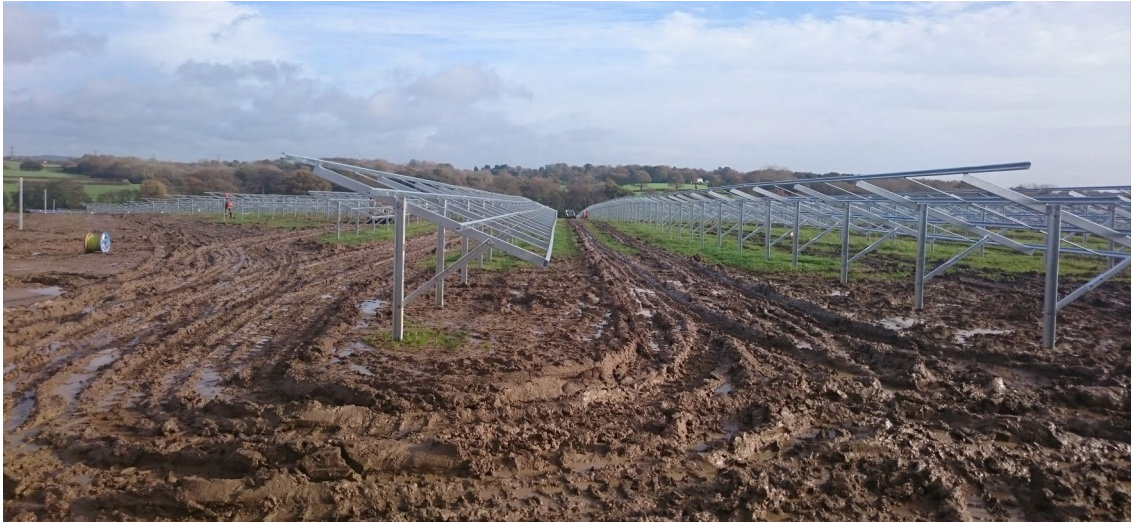
Inserts 36 and 37: Winter Installation (2015) and Operational Site (2022)
